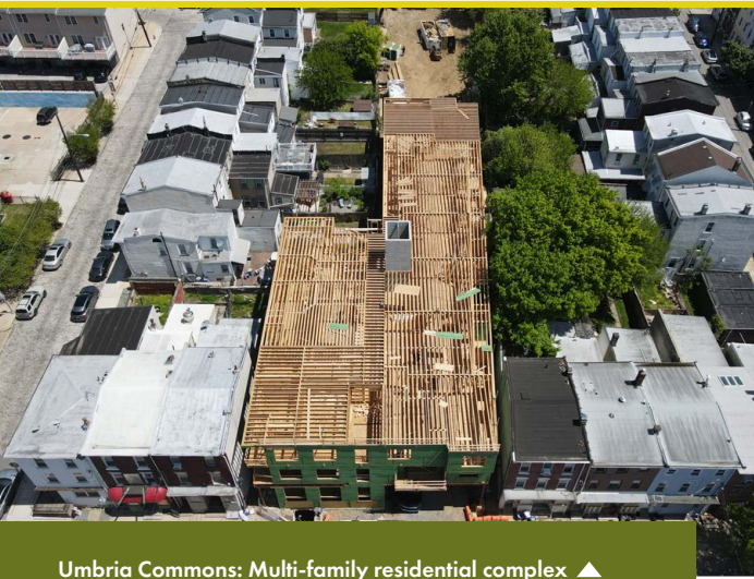
Umbria Commons: Multi-family residential complex ▲ under construction in a compact site in Philadelphia
